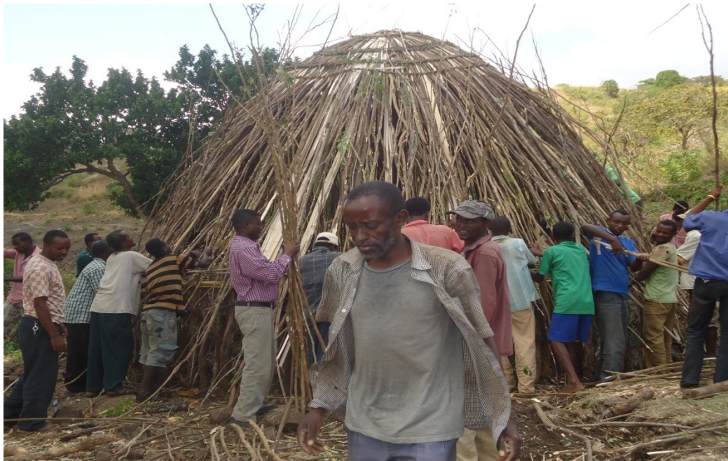
Ganta Idir association including: mala, lathi and ayle, constructing a house for mala widow. Photo by Boshia B. April 2013
